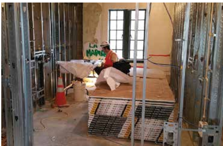
The College Principal's quarters include a modest kitchen. Here you can see initial framing has been completed and plumbing laid in.
