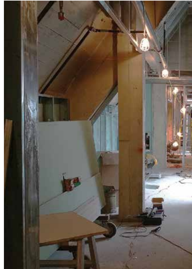
The apartment for the College Dean is being fashioned from a former UC maintenance storage room. It features three new skylights to provide natural light to what will be a truly unique place to live.
