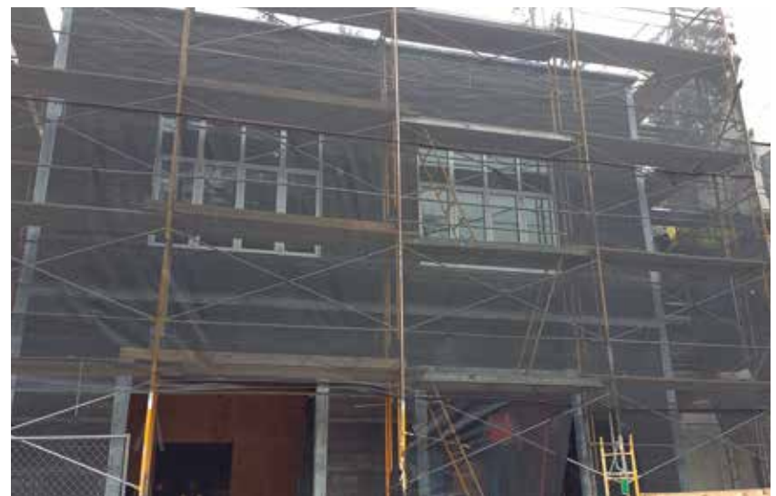
The first floor of the annex will serve as a kitchen storage and utility area; the second floor features an expansive game room. Outer walls will match the historical features of the rest of the Hall.
